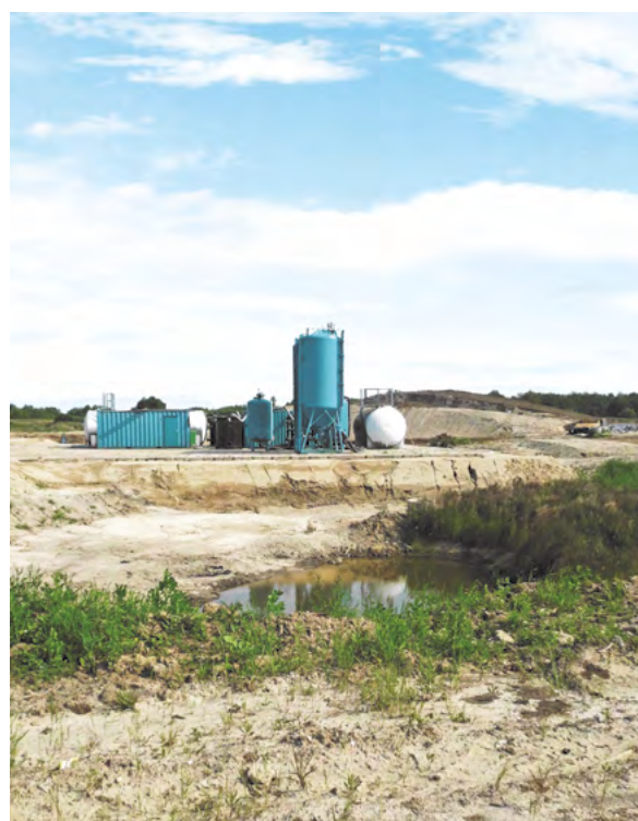
Figure 34: Groundwater treatment system; Source: Construction and real estate authority, Mecklenburg-Western Pomerania, Federal Construction Division
