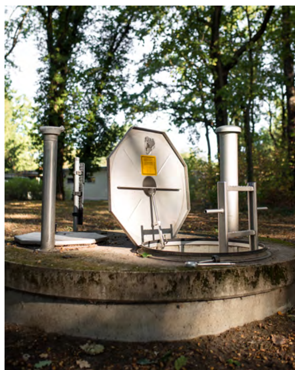
Figure 18: A deep well on the premises of a Bundeswehr site; Source: Bundeswehr/Jenny Bartsch
