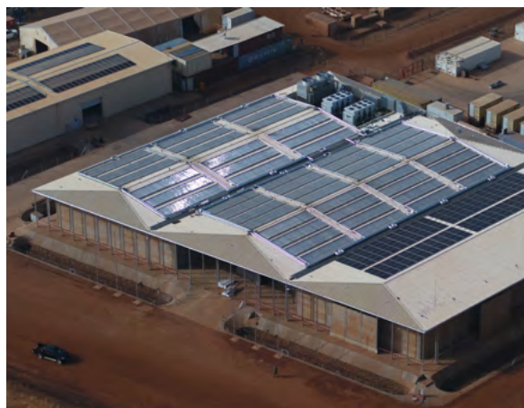
Figure 16: Photovoltaic system in the Gao/Mali field camp; Source: Bundeswehr/Marc Vigansky
